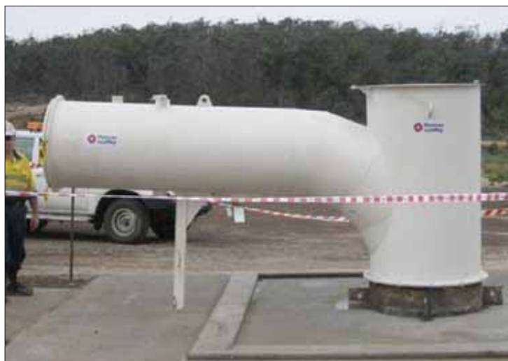
Figure 33.6: Inertisation connection facilities
