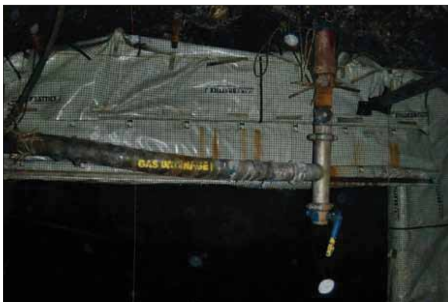
Figure 9.5: Bottom of gas riser at entrance to the FAB
