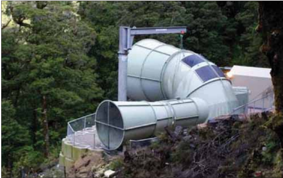
Figure 8.5: The surface back-up fan
