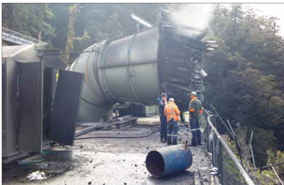
Figure 8.10: The surface fan after the first explosion
