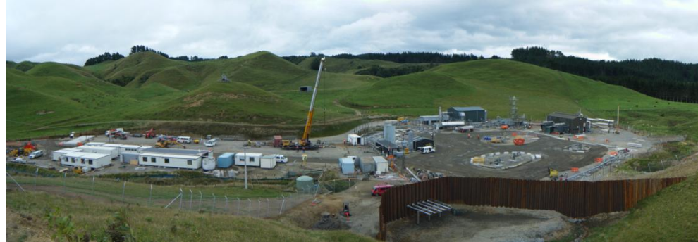
Ahuroa gas storage project
