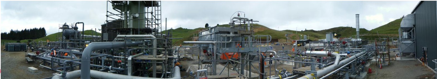
Ahuroa Gas Storage Stage 1
